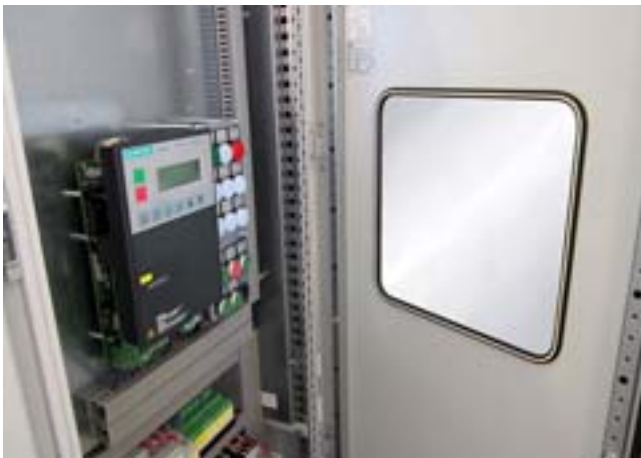
M19 Example of window in door for viewing internal display
